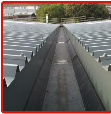
FRP ROOF GUTTER
