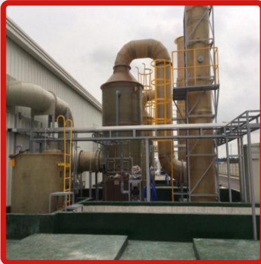
PP FRP SCRUBBER SYSTEM
